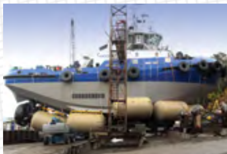
Draft reduction for newly constructed tugboat launching using Salvage Pontoons 40,000 lbs. and Salvage Pontoons 70,000 lbs.
