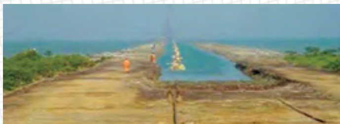
Installation of oil pipeline in the Middle East using Salvage Pontoons 6,000 lbs.
